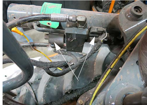
Lock Valves -Typical View
