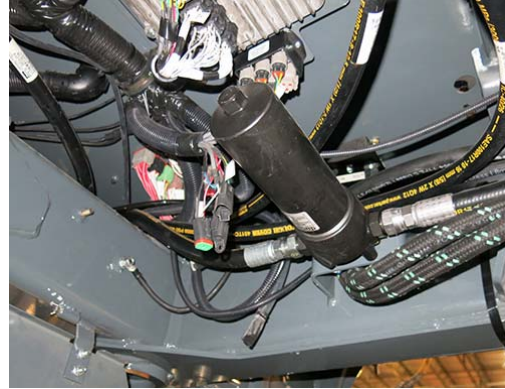
Pressure Filter (Located beneath right-hand side of machine - lower metal shield to access) -Typical View
