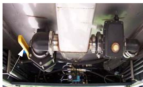
Sump Valve (Located beneath the solution tank) -Typical View
