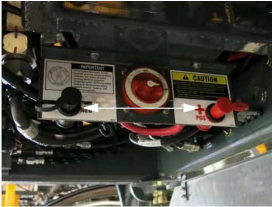
Auxiliary Battery Charging Posts (Located beneath center of machine) -Typical View
