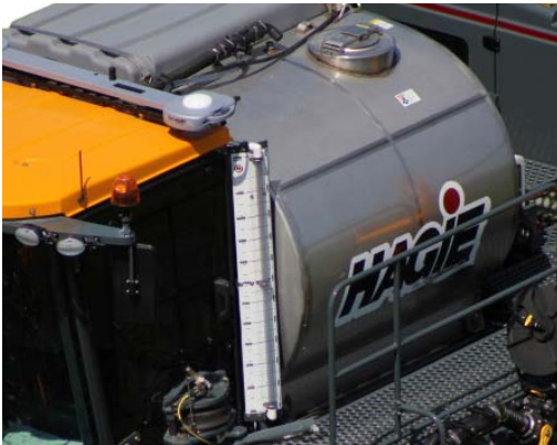
Solution Tank -Typical View
