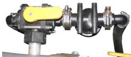
Rinse Tank Supply Valve (Located on the rinse tank) -Typical View
