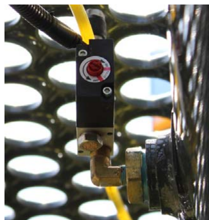
Pilot Valve (Located beneath catwalk on left-hand side of machine) -Typical View
