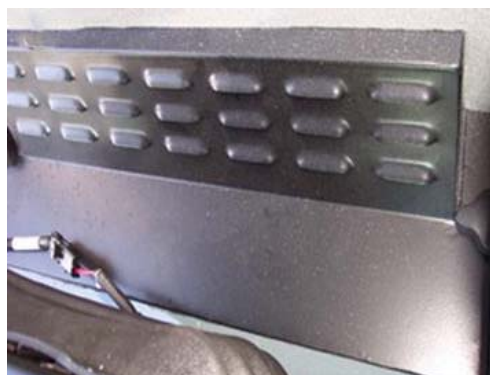
Fresh Air Filter Access Panel -Typical View
