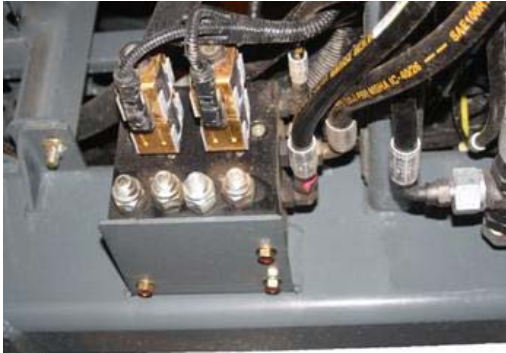
Valve Block (Located on the underside of machine) -Typical View
