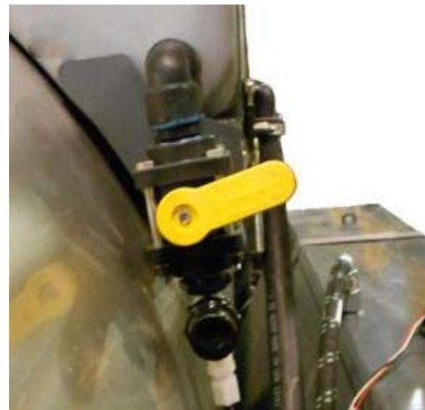
Foam Marker Hand Valve (Located near the rear of Rinse Tank) -Typical View
