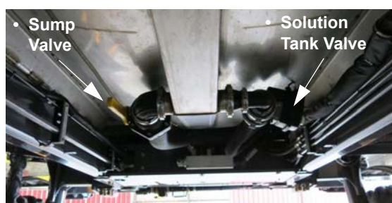
Solution Tank and Sump Valves (Located beneath the solution tank) -Typical View
