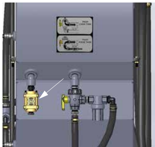
Tank Drain Valve -Typical View
