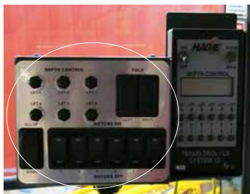
Detasseling Control Panel -Typical View
