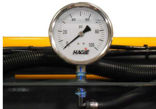
Pressure Gauge -Typical View
