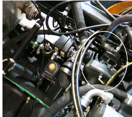
Solution Pump (Located near center of machine) -Typical View
