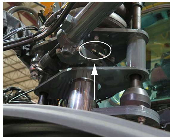
Collar Grease Zerk (4) (Located beneath each air bag mounting plate) -Typical View
