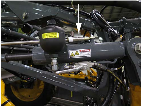
Position Sensor -Typical View
