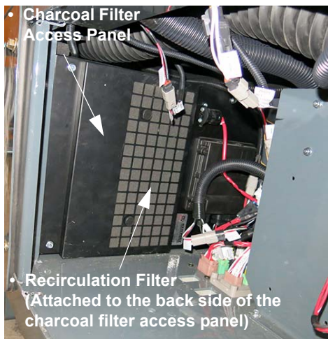
Charcoal Filter Access Panel (Located behind exterior service panel on right-hand side of cab) -Typical View
