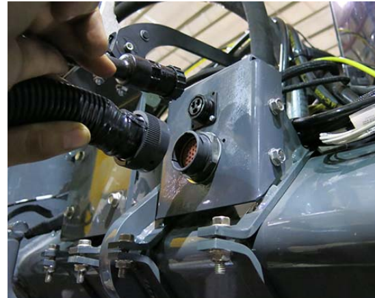
Electrical Connections (Right-hand side of machine shown) -Typical View
