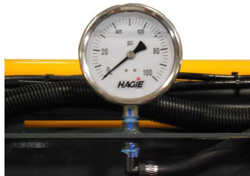
Pressure Gauge -Typical View
