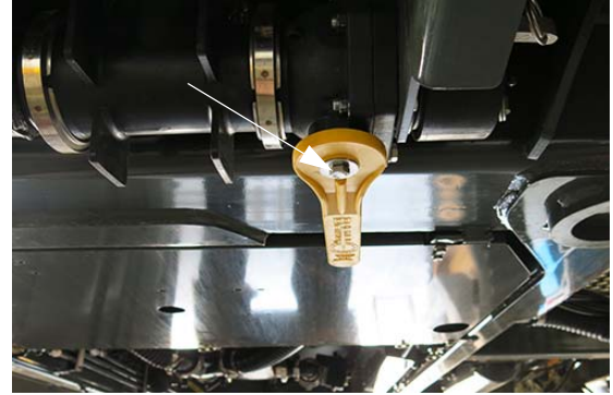
Front Fill Valve Bolt -Typical View
