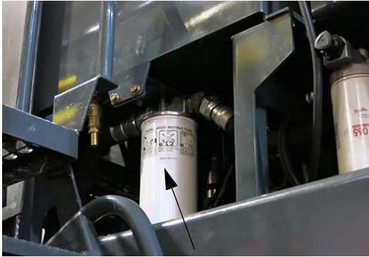
Case Drain Filter (Located on left-hand side of machine) -Typical View
