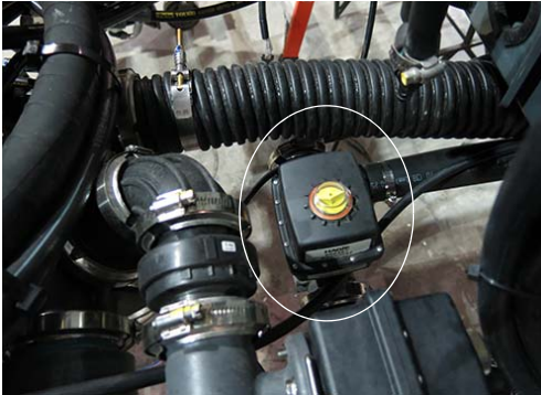
Agitation Valve (Located near center of machine) -Typical View * View shown from top of machine
