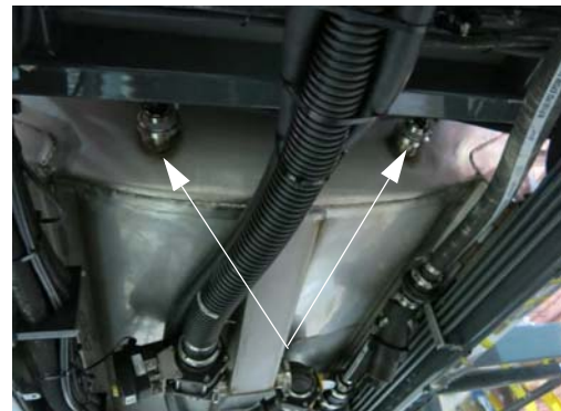
Jet Agitators (Two located on each end of solution tank) -Typical View
