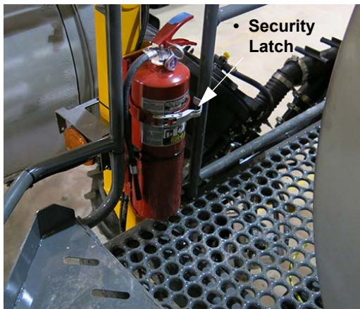
Fire Extinguisher (Located along the catwalk on left-hand side of machine) -Typical View
