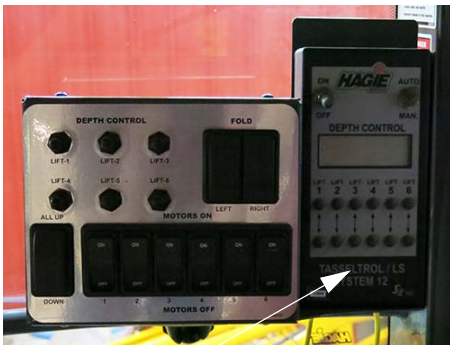
Tasselrol Control Panel -Typical View
