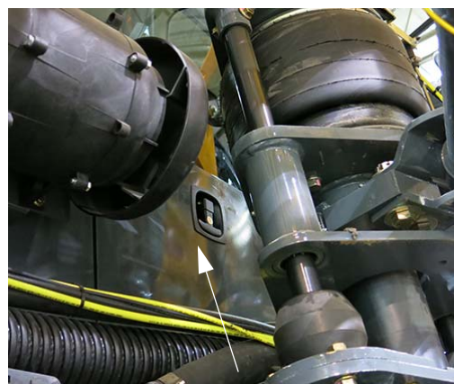
Exterior Service Panel (Located on right-hand side of cab) -Typical View
