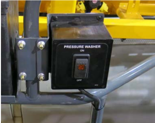
Pressure Washer Switch (Located along the handrail on left-hand side of machine) -Typical View
