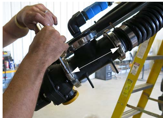
Front Fill Manifold Clamps -Typical View
