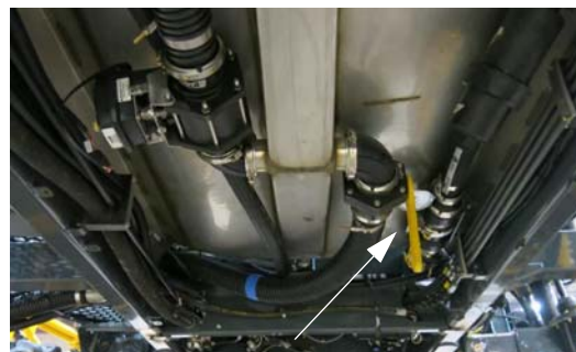
Sump Valve -Typical View
