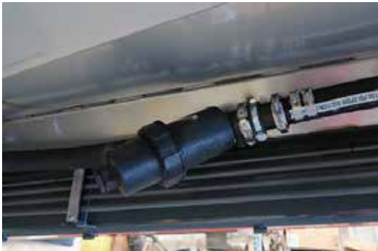
Solution Line Strainer (Located beneath the center right-hand side of machine) -Typical View
