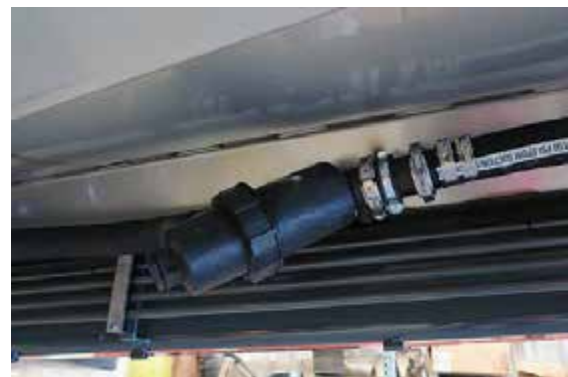
Solution Line Strainer (Located beneath the center right-hand side of machine) -Typical View
