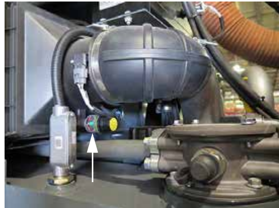
Filter Minder (Located near engine pre-filter - open hood to access) -Typical View
