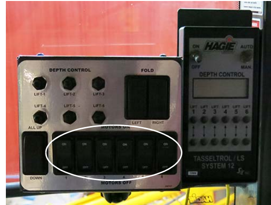
Motor Control Switches (Located on the detasseling control panel) -Typical View
