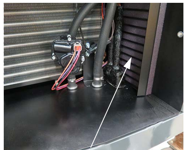
Recirculation Filter (Located along the right-hand side of service compartment) -Typical View
