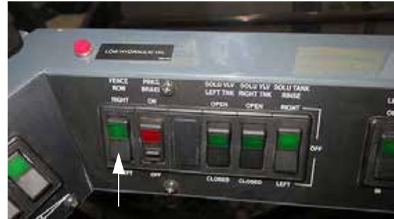
Fence Row Switch (Located on the side console) -Typical View
