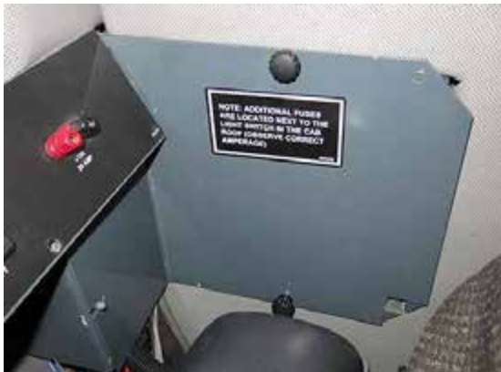
Fuse Panel (Located on the right-hand side of the operator’s seat) -Typical View
