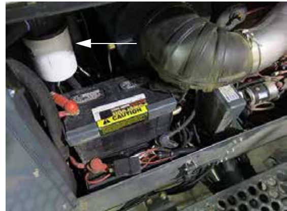
Hydraulic Suction Filter (Located behind right-hand engine compartment) -Typical View
