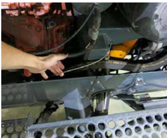
Tank Drain Valve -Typical View
