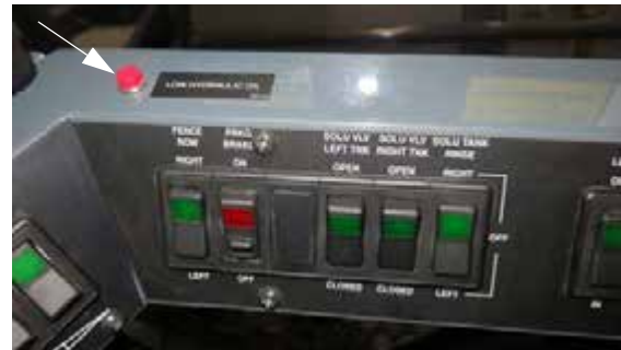
Low Hydraulic Oil Indicator (Located on the side console) -Typical View
