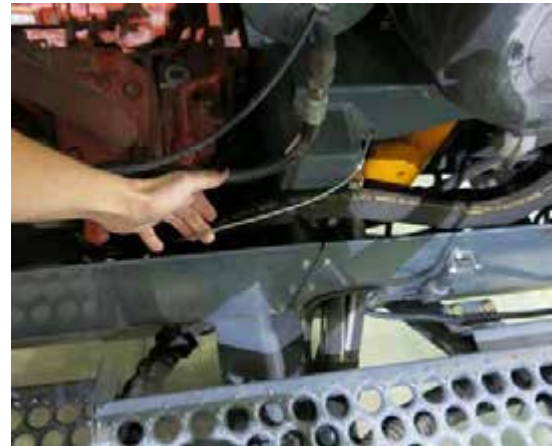
Tank Drain Valve -Typical View
