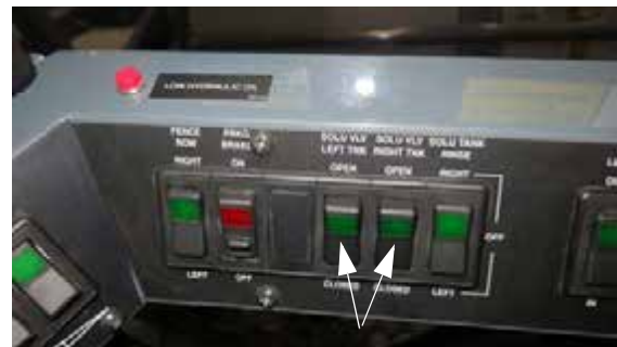
Solution Tank Valve Switches - Left/Right (Located on the side console) -Typical View
