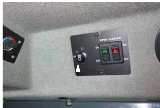
Highway Lights Switch (Located on cab headliner) -Typical View
