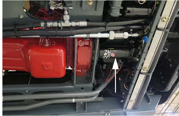
Charge Pump Filter (Located beneath rear of machine) -Typical View
