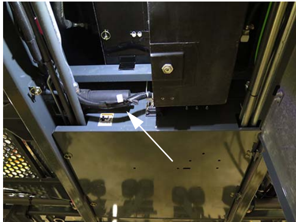
Pressure Filter (Located beneath center of machine) -Typical View
